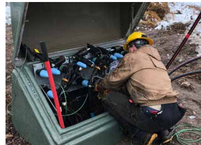
A cabinet with both the old cable and new cable is prepped on Washington Island.
