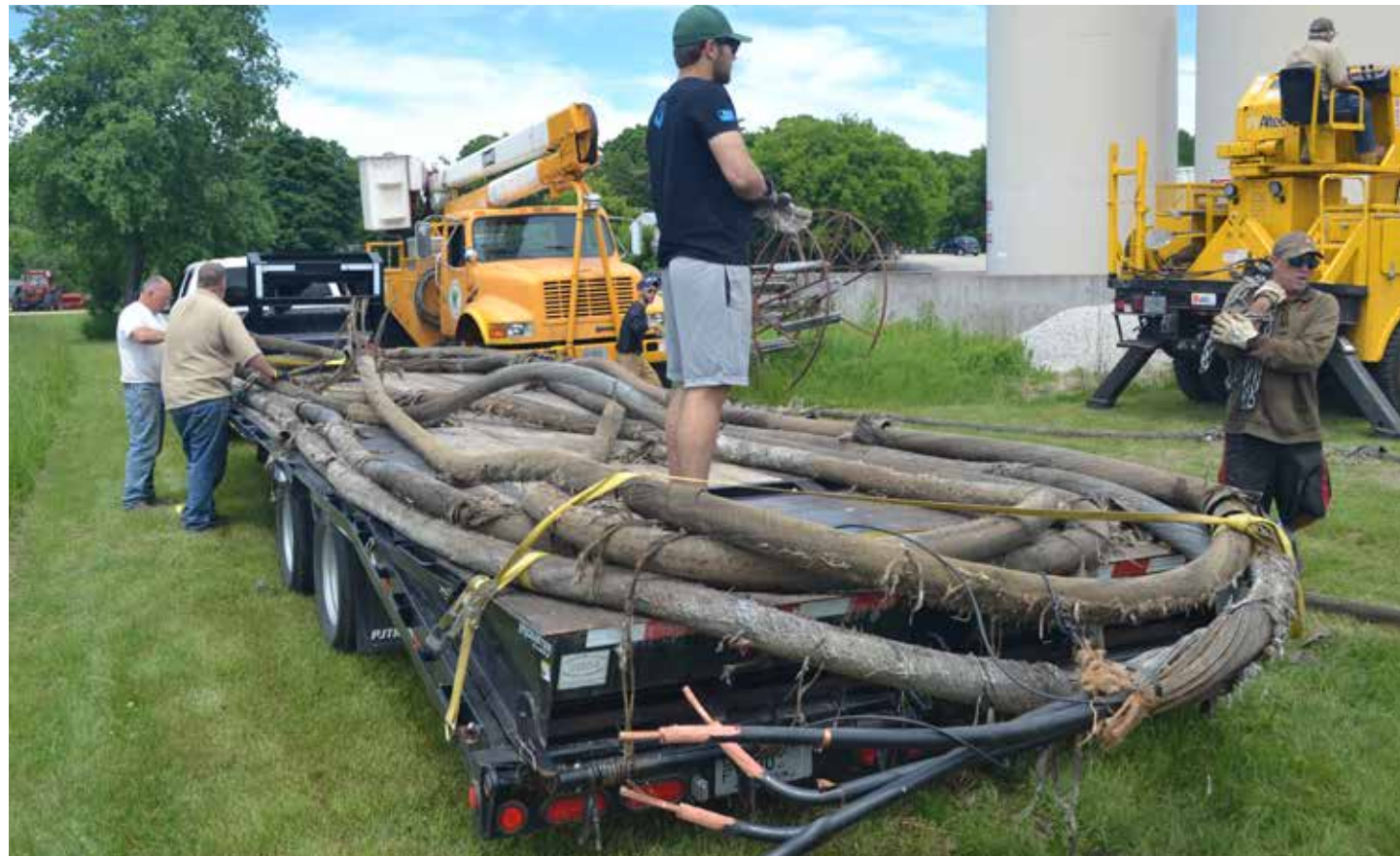
Leftover cable from the original 1981 power cable installation was used as a temporary replacement for a section of failed cable.
