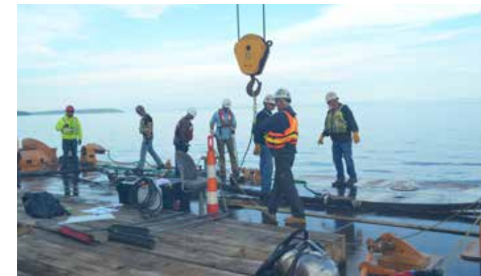
Contractors prepare to return spliced/repared cable to the bottom of Death’s Door Passage.
