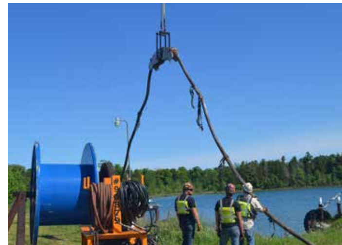
Workers wind leftover cable on a reel to take out for the temporary repair.
