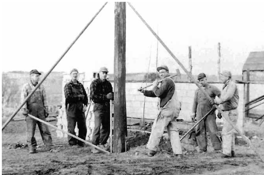
Circa 1946 photo of workers "planting" a power pole along the East Central Electric service line.
