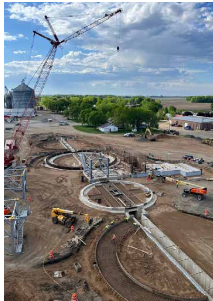
As part of the project, grain bins are being moved to new foundations, pictured under construction.
